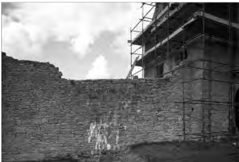
Pl. 3.27—Pre-conservation view of the exterior eastern façade of the south-eastern bawn wall (Photographic Unit, NMS).
