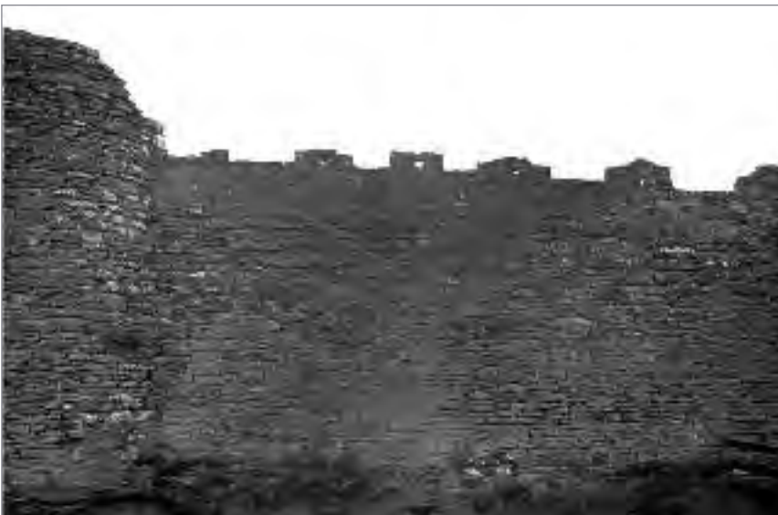
Pl. 3.23—Pre-conservation view of the western bawn wall next to the north-west corner tower (Photographic Unit, NMS).
